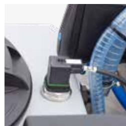
Fill level sensor in the tank
