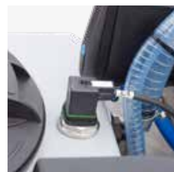
Fill level sensor in the tank
